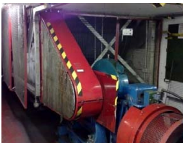
Figure 15.1 Chain driven Escalator monitored by MCM
