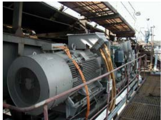
Figure 6: Conveyor Drive Motor
